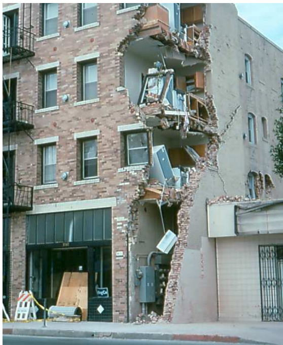
Earthquake losses add up in both lives and property damage.
