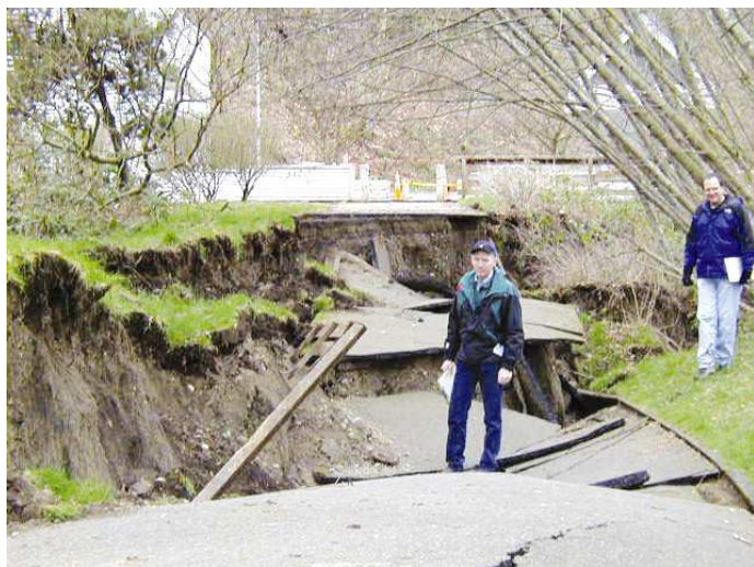
Earthquake damage affects roads, telephone systems, water systems, and other critical services. This image shows damage from the Nisqually Earthquake in Washington, 2001).
