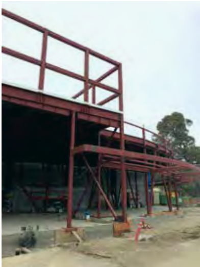
Construction is underway on the expansion of Contra Costa College's new Physical Education/Kinesiology complex featuring a renovated gymnasium and a modernized Gym Annex.
